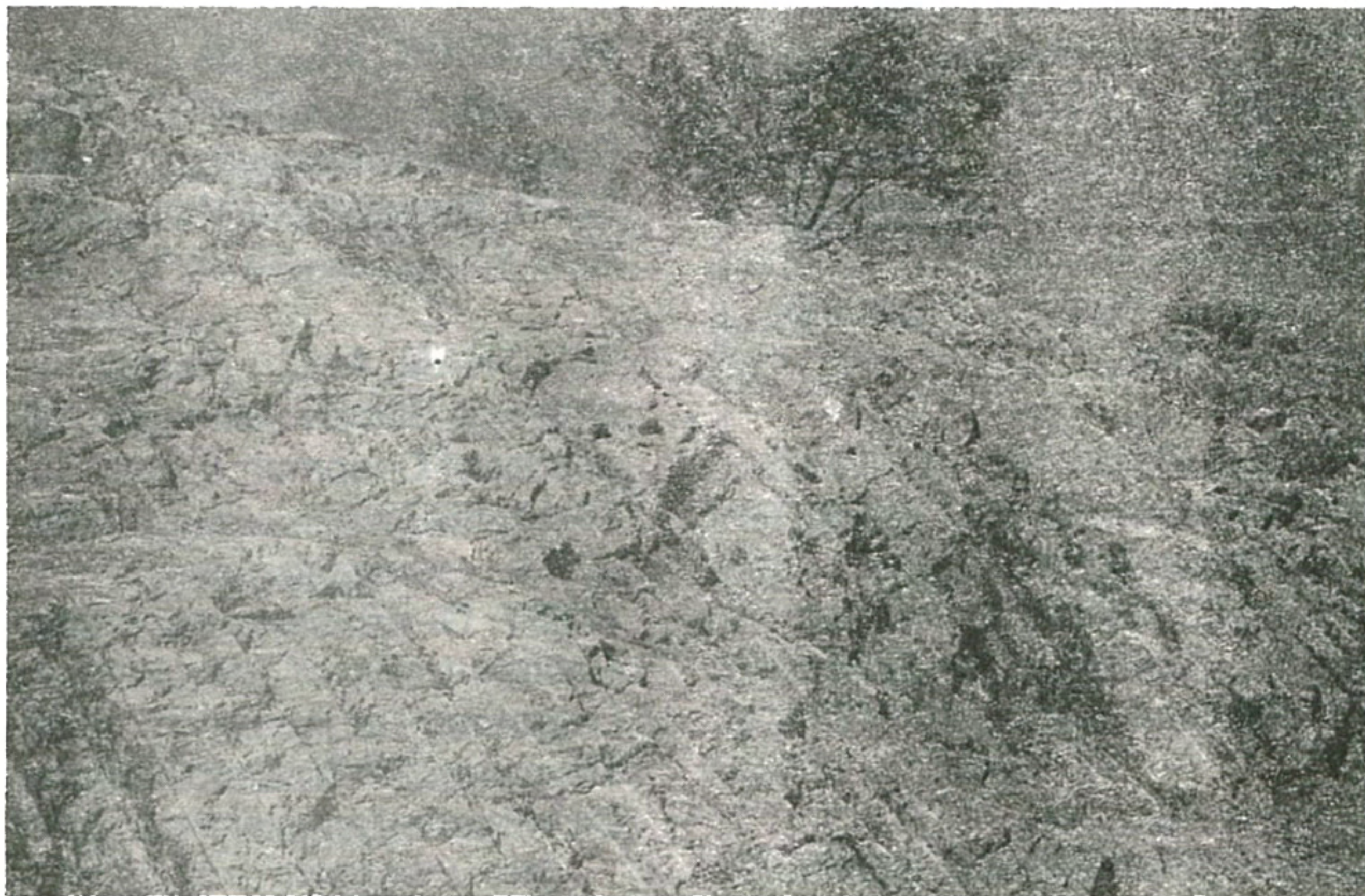
Photo 2. The Faces of Slope cutting have done by split blasting method. In this photos can be seen the type of plane failure and rock fall.
