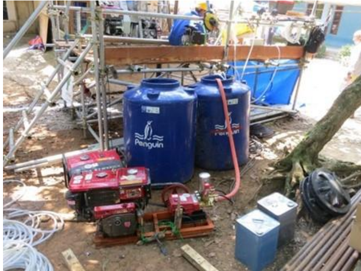
Figure 12 - Photograph of pump setting
