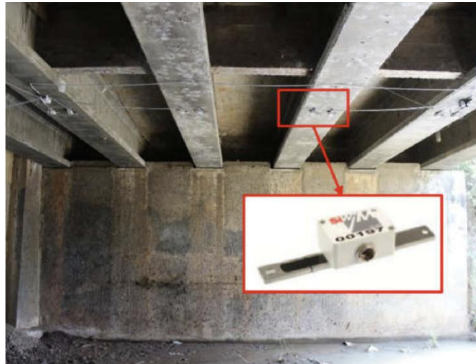
Fig. 1 B-WIM instrumentation on the Pawiro Baru Bridge (Nugraha, Sidi, et al., 2023)
