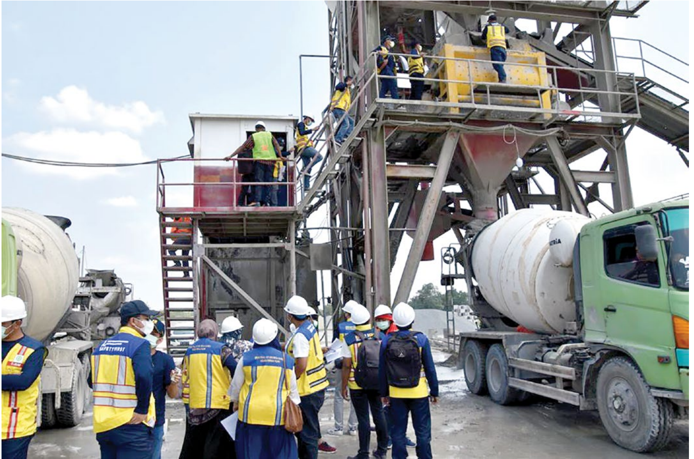
Kunjungan ke Controlling Room Batching Plant .
